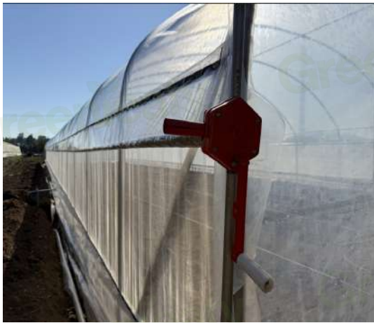
Two sides ventilation system
