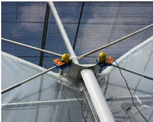
Top ventilation system
