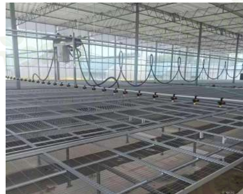
Strip sprinkler irrigation
