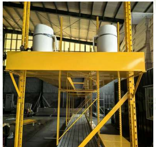
Ventilation system for grow rack
